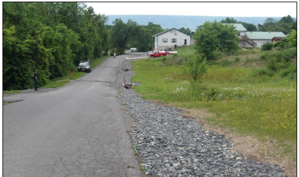
Top center: Old Butchershop Road, Fermanagh Township. 3 cross pipes and 333 feet of underdrain. Page 4 left: Maze Road, Delaware Township. 3 turn outs, 12 cross pipes, 1,281 feet of geo fabric, and 769 feet of underdrain Page 4 right: Cider Press Road, Beale Township. 1 new cross pipe to better improved drainage.
